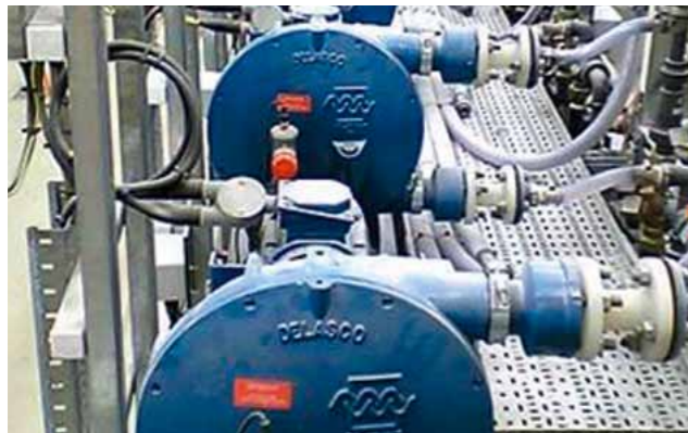
PAX and flocculants - DL45 pumps (Gold mining)
