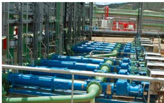
Mineral Pulp - 24015 pumps delivering 130m³/h each (Nickel mining)
