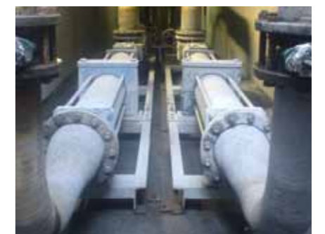
Clay sludges – 240ID5 pumps
