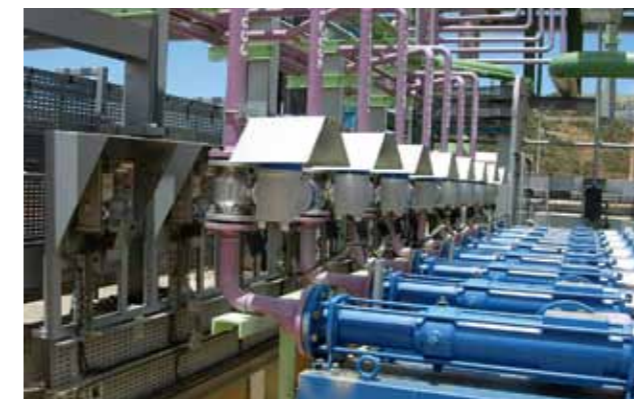
Diluted Flocculants 2515 pumps for 2 to 6m³/h (Nickel mining)
