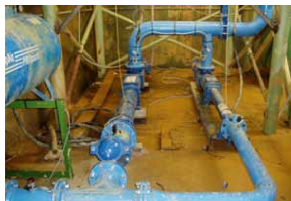
Filter press feeding: one high flow rate pump and one high pressure pump
