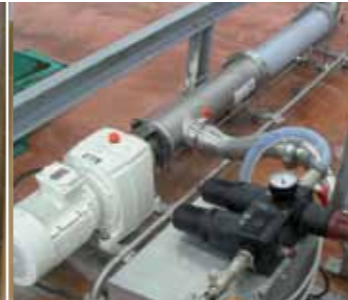
Wine filtration skid
