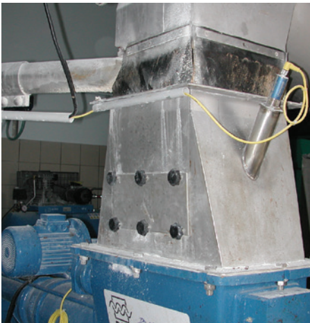
Level control built into a control box.
