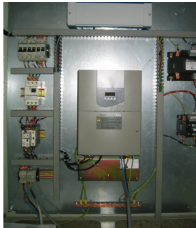
Level control in lime treatment applications.
