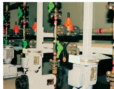
Ferric chloride pumping in purification station.
