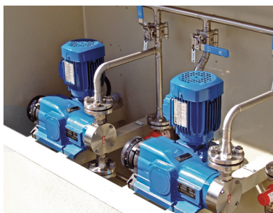
Sulfuric acid metering in mining
